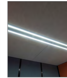
DUAL LED STRIP LIGHTING integrated into facilities arch
